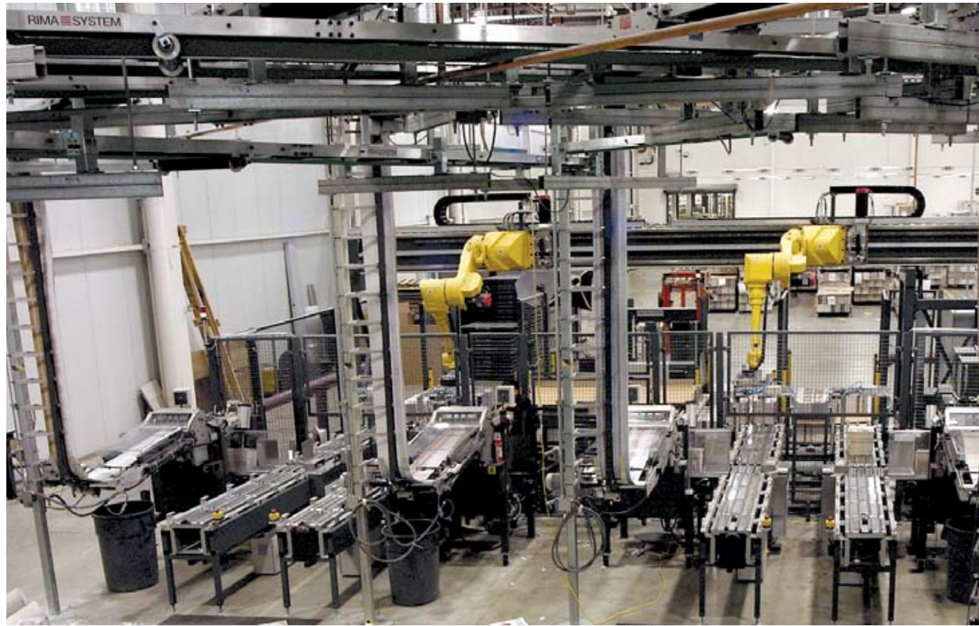
▲ View of the stacking and palletizing area with four overhead lines, four RS 50S stackers, four stack conveyors with manual stack pick-up for samples and the RS 500 Double Palletizer.
