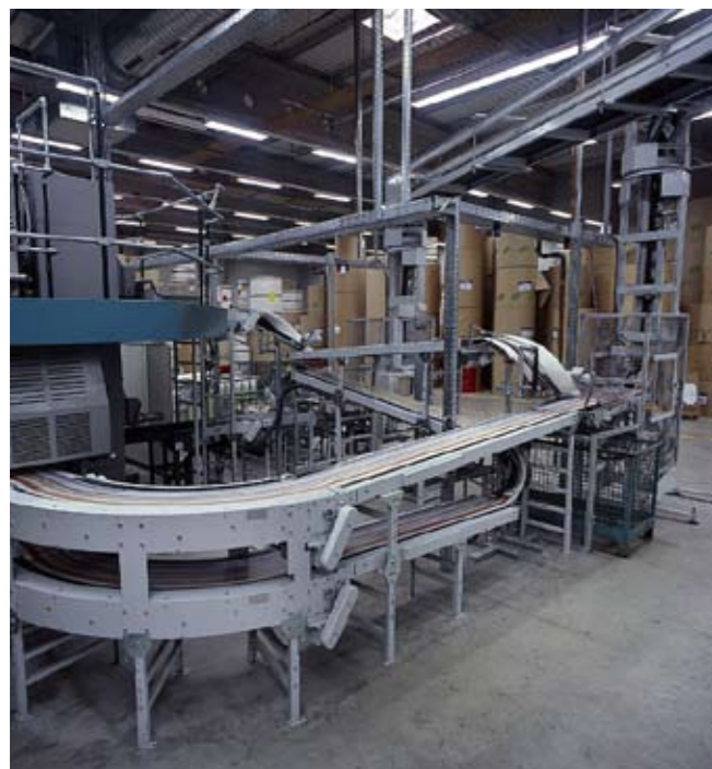
The floor conveying systems transport the shingled stream from the four press deliveries to the pick-up stations of the overhead conveyor system.
